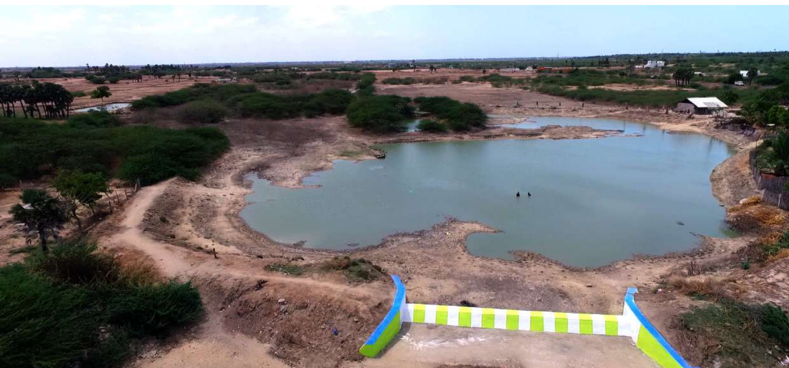
Check dam Constructed at Thathanenthal rivulet in Thathanenthal panchayat of Thiruppullani block
