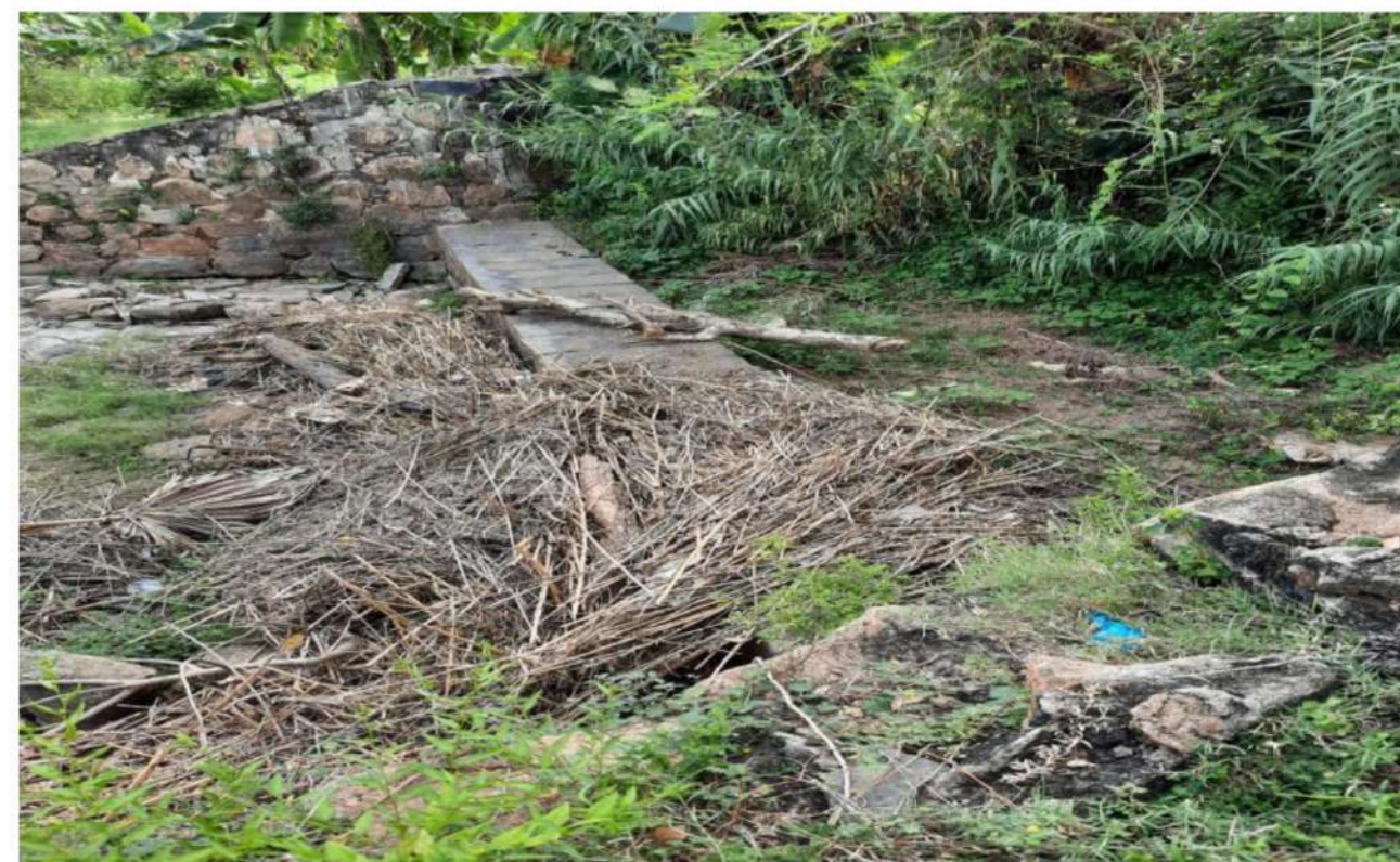
Hydrological problem - Vellore anicut requiring renovation
