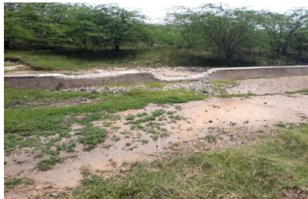
Hydrological problems in Varavani Tank Weir Partially Broken: Water is not stored to its full capacity. Hence the quantity of water supplied to irrigation is getting reduced. Rectification to this work is of minor in nature and should be carried out immediately.
