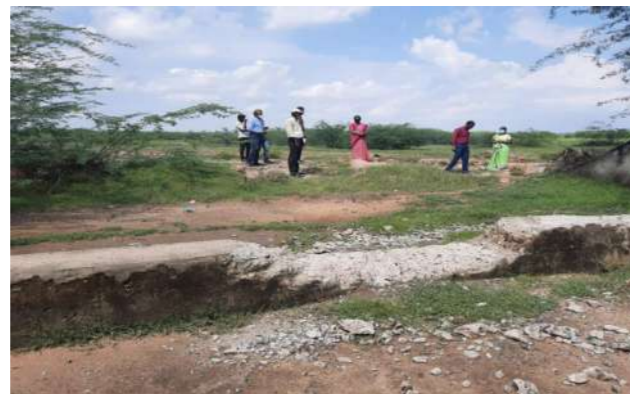
Hydrological problem is no defined course in weir of Varavani tank: Surplus water going through field. Action to be initiated for forming a course for the smooth and efficient flow of water to the lower tank.
