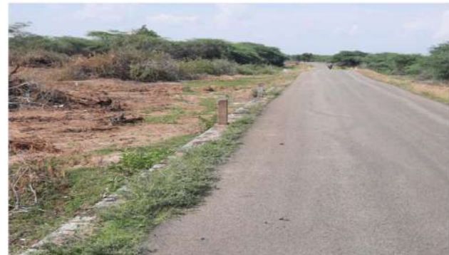
Hydrological problem in Suriankottai river: Lot of encroachment and river flowing as two compartments. Action to be taken is to remove encroachment.
