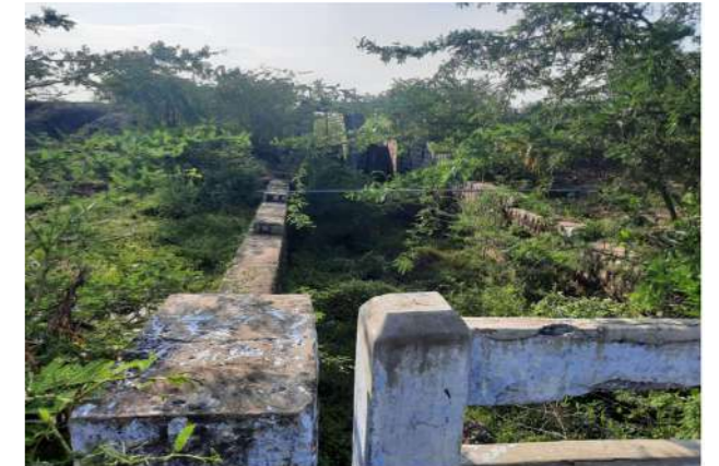
Hydrological problem- Head Sluice for R.S. Mangalam tank in dilapidated condition and Renovation works need to be taken.
